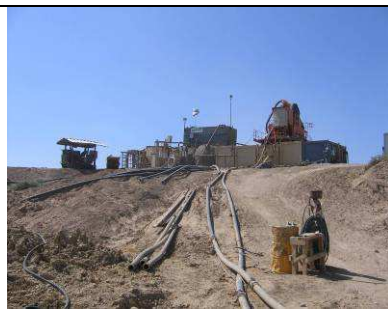
Figure 15 - Station de bentonite
